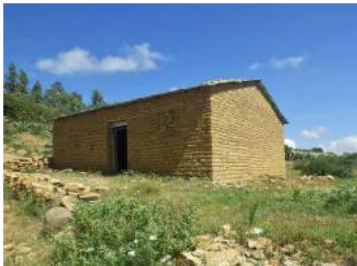
Fig. 23: The mosque entrance. Note the two blocked windows and the potholes in the façade.
